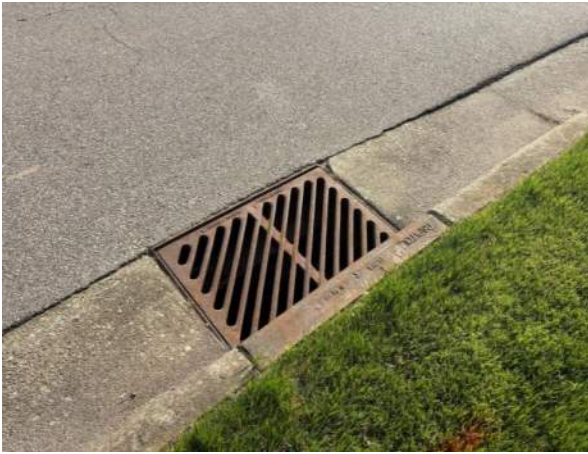
Representative photo of water infrastructure along Paramount Parkway.
