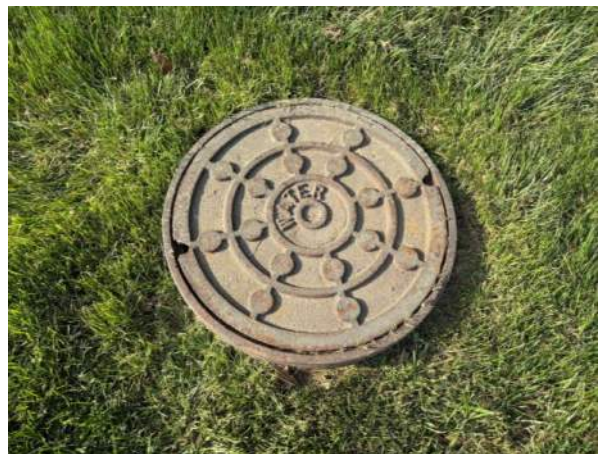
Representative photo of a storm drain located along Paramount Parkway adjacent to the Subject Property.
