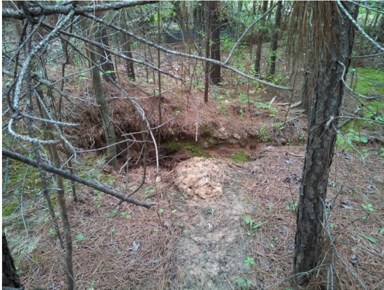
Photo 15 Outfall 1-10 dam failure
