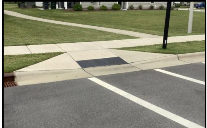
Deficient Curb Ramp (Slope)
